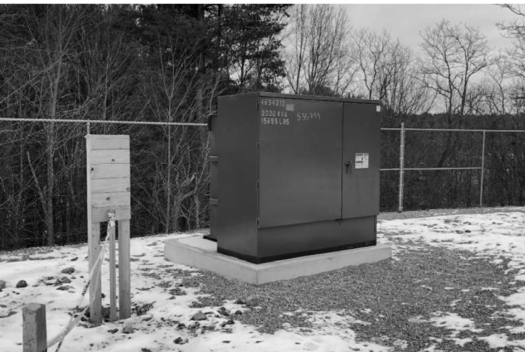
View of electrical transformer at west side of the site
