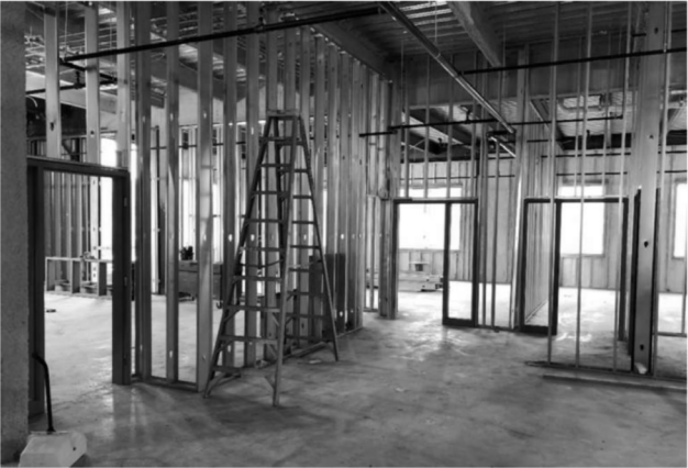
View of interior partition framing and hollow metal door frames at Second Floor
